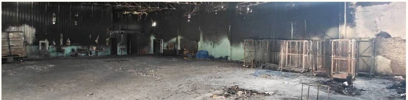
Inner walls of the warehouse covered with black soot and other burnt materials.
