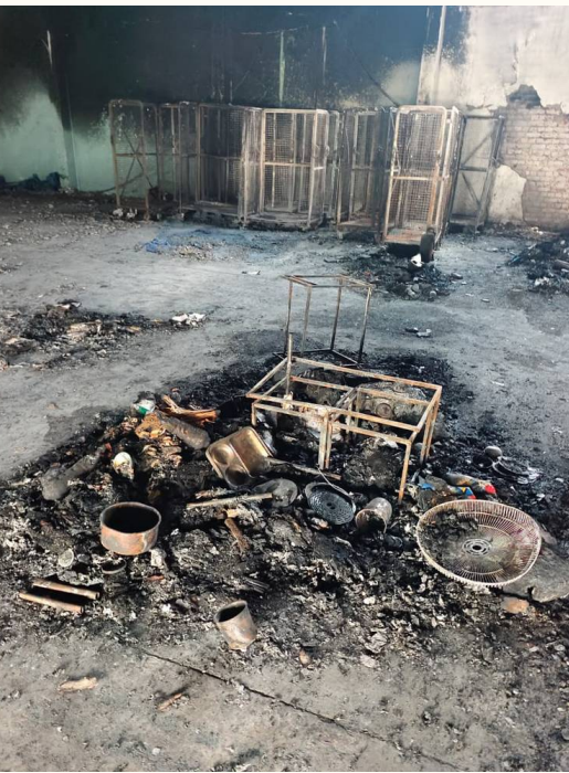
Walls of the Amazon warehouse covered with black soot and other burnt materials.
